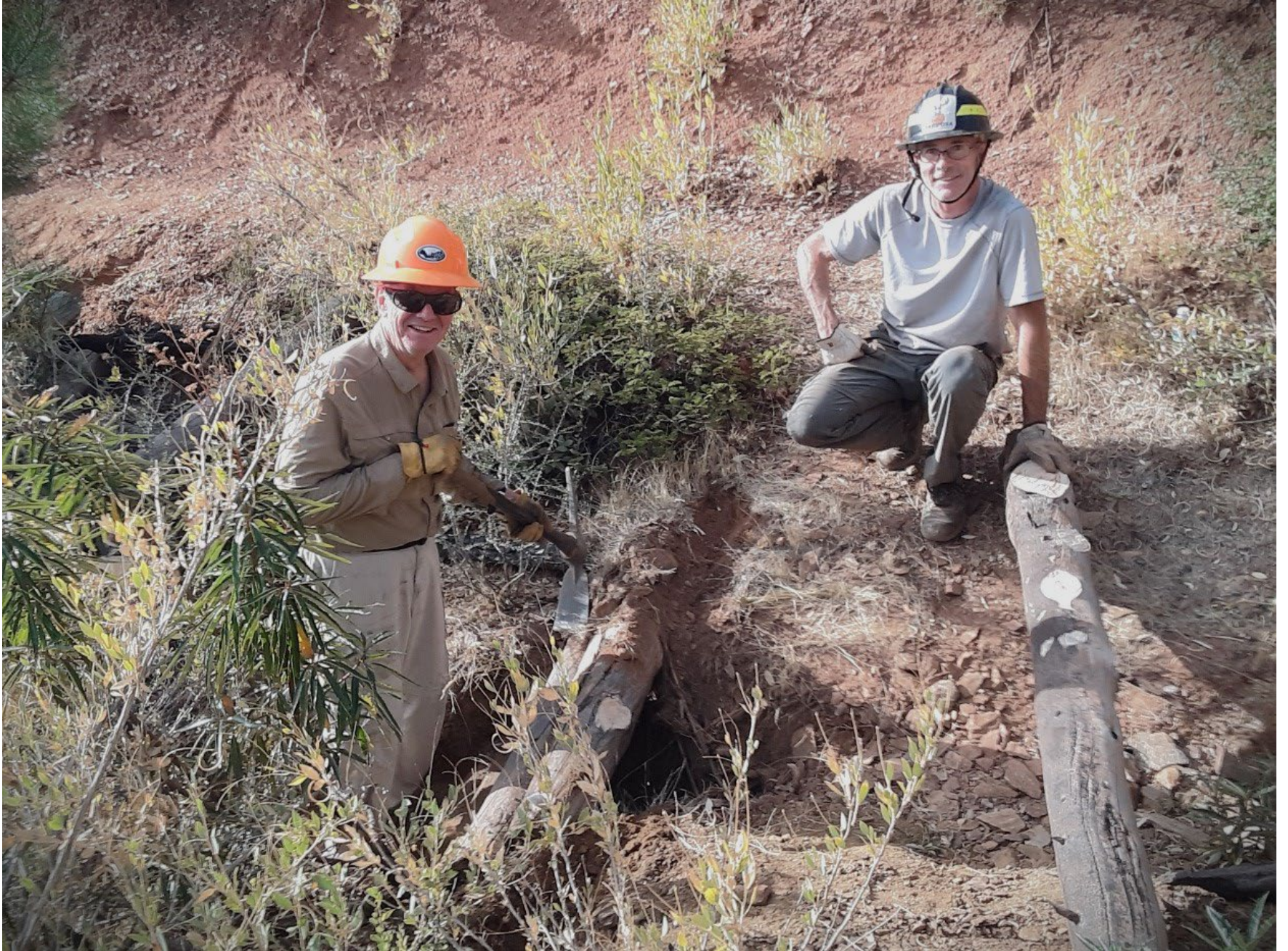
Paul and Bill building retaining walls at gully washouts along the Savage-Lundy Trail
