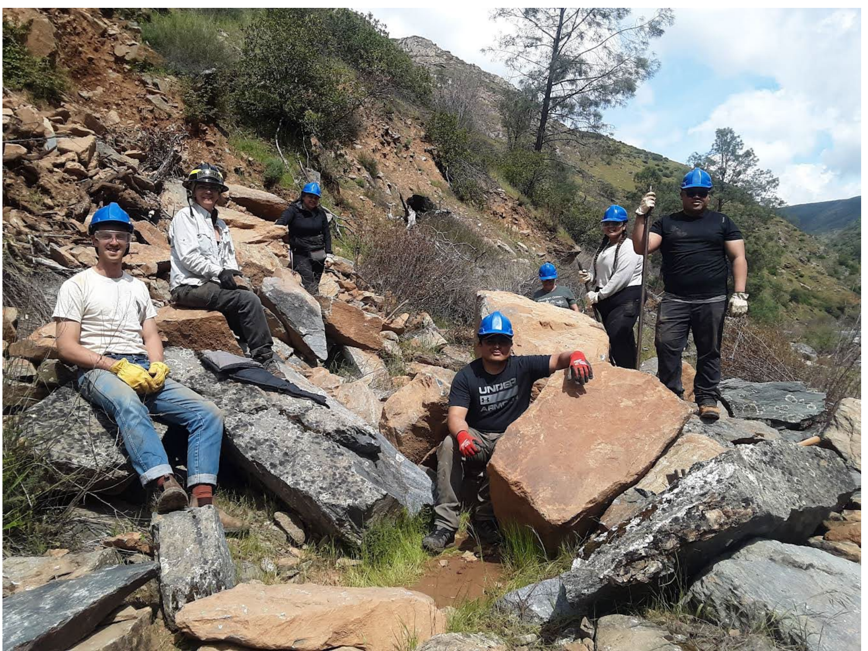
A volunteer crew clears a path through a rockslide on the Merced River Trail
