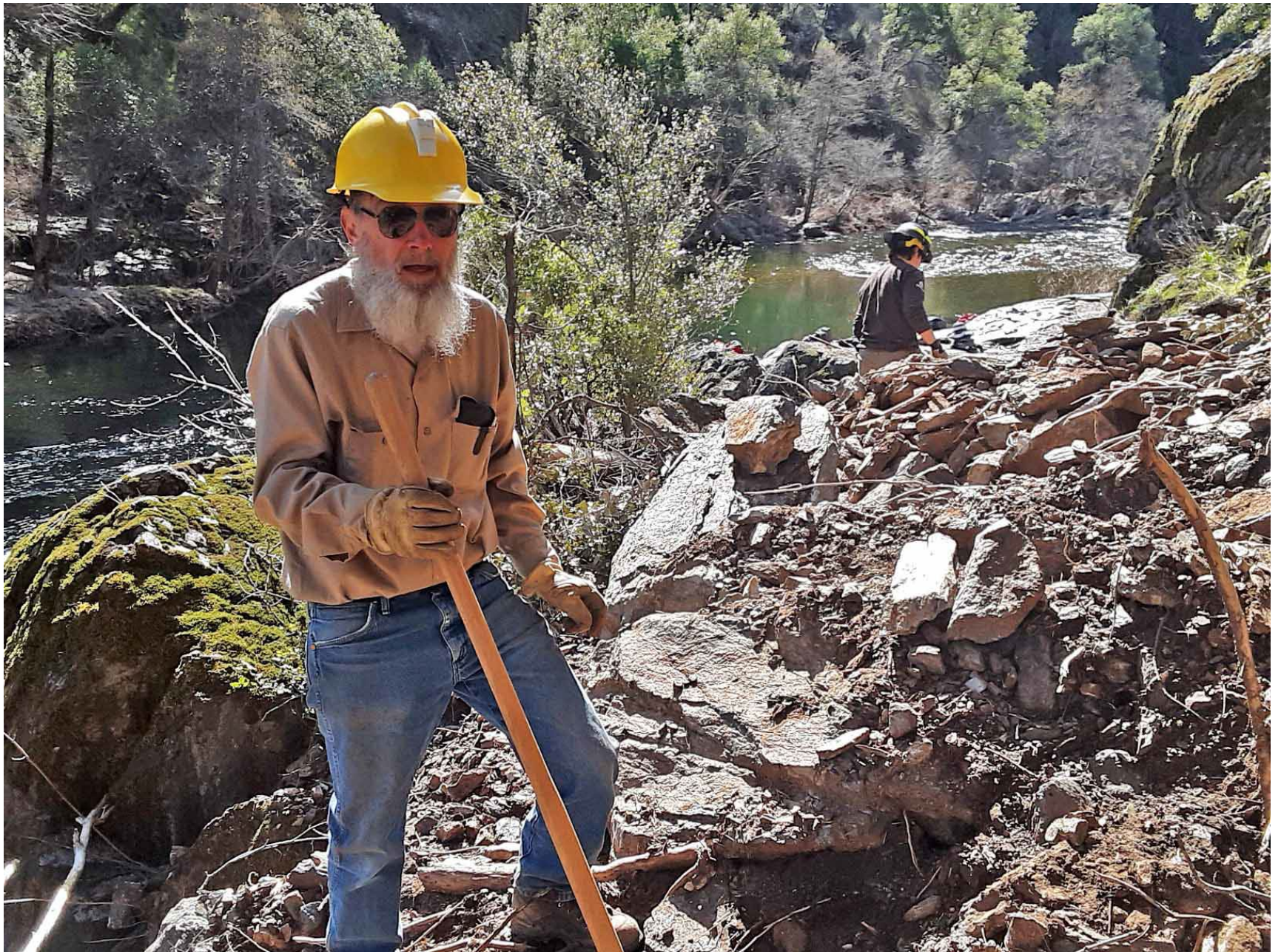
Steve working with 8-person crew to clear a big rockslide on the Hite's Cove Trail
